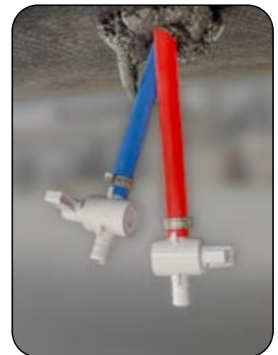
Low-Point Drain Valves located under the RV
