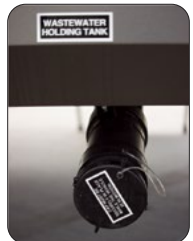
Sewer Outlet Connection Is Located Under the RV on the Off-Door Side
