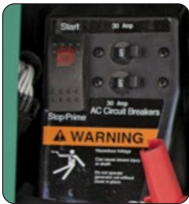
Generator main power & circuit breaker switches.
