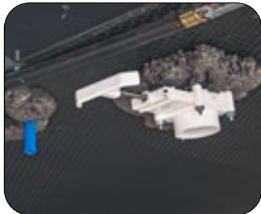
The Fresh Water Holding Tank Gate Valve is located under the RV
