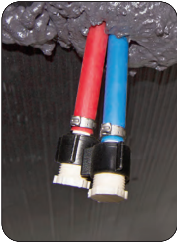
Low-Point Drain Valves located under the RV
