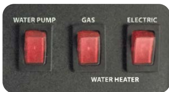
Water Pump & Water Heater On/Off Switches
