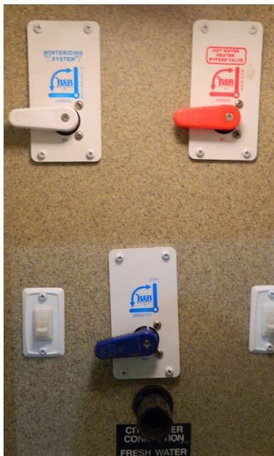
Typical valve positions for gravity water fill usage (connect hose to black inlet)
