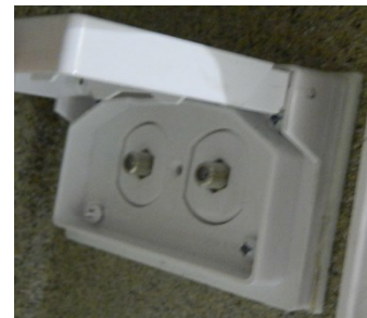
Typical cable/satellite outlet:
