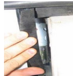
Step 2 – Typical Schwintek motor location, viewed from inside the RV.
