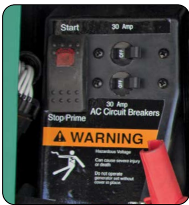
Generator main power & circuit breaker switches.
