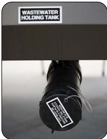
Sewer Outlet Connection Is Located Under the RV on the Off-Door Side
