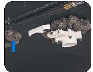
The Fresh Water Holding Tank Gate Valve is located under the RV
