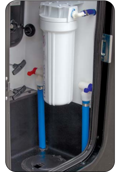
Water Filter and Low-Point Drains are located in the Universal Docking Station
