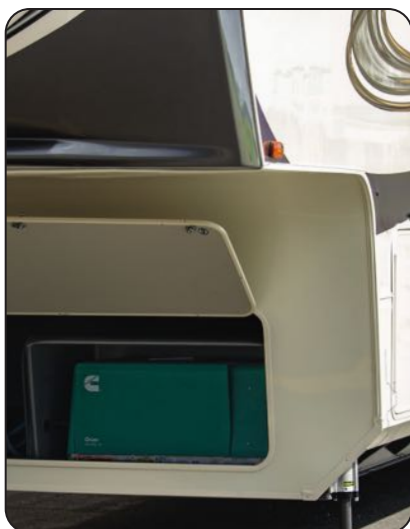
Generator (if so equipped) is located in the front compartment of your RV.
