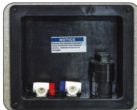
Hot & Cold Water Washer Hookups are typically located in the front bedroom or in the rear garage area.
