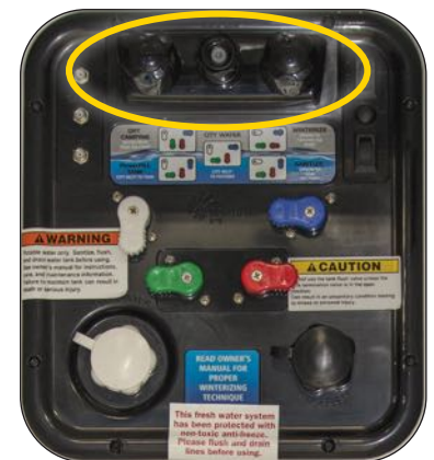
Exterior Spray Port
