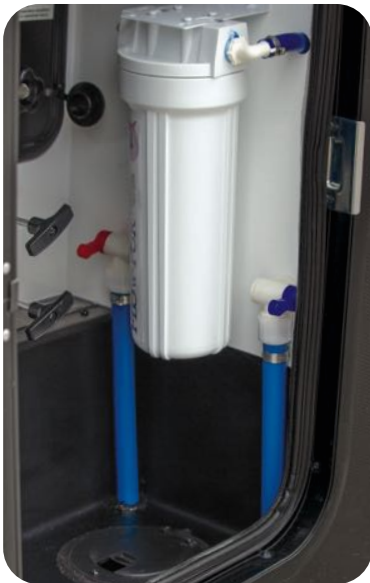
Low-Point Drains are located in the Universal Docking Station
