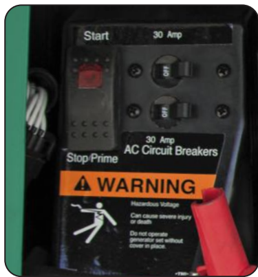
Generator main power & circuit breaker switches.
