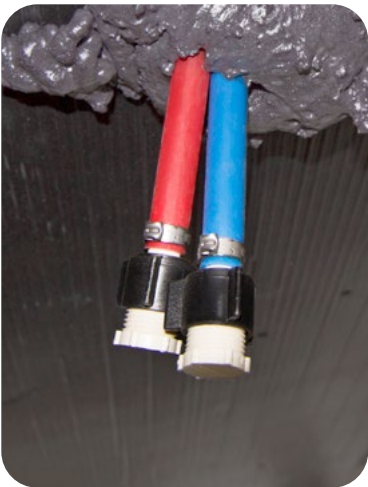
Low-Point Drains located under the RV
