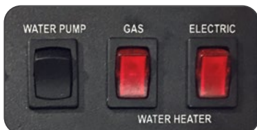
Water Pump & Water Heater On/Off Switches
