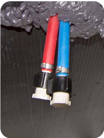
Low-Point Drains located under the RV
