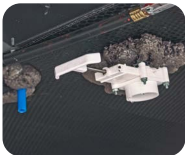
Fresh Water Holding Tank Gate Valve, located under the RV
