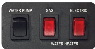
Water Pump & Water Heater On/Off Switches
