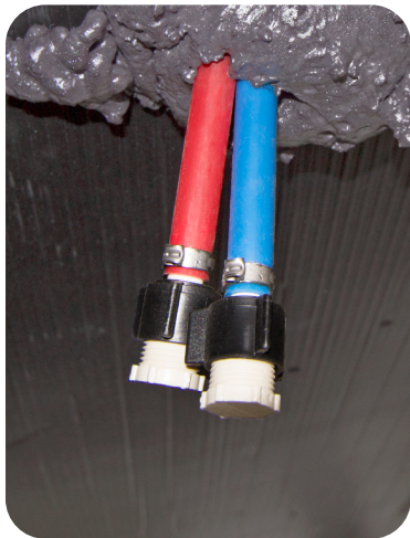
Low-Point Drains located under the RV
