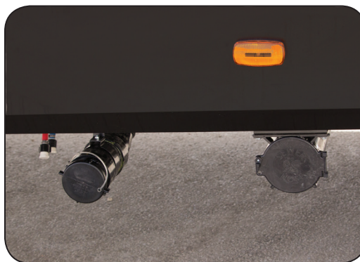
Sewer Outlet Connections are Located on the Off-Door Side
