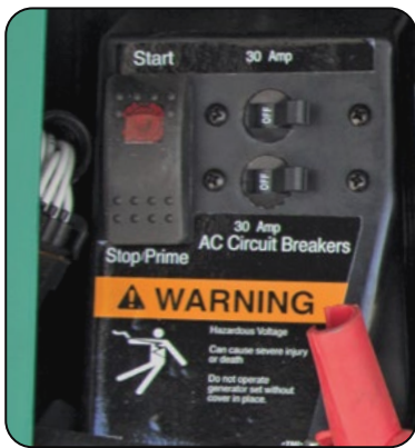
Generator main power & circuit breaker switches.
