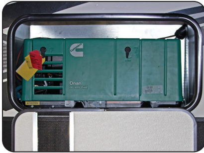
Generator (If So Equipped) Is Located in the Forward, Off-Door Side Compartment of the RV.
