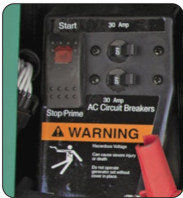
Generator main power & circuit breaker switches.
