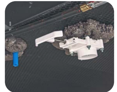
Fresh Water Holding Tank Gate Valve, located under the RV
