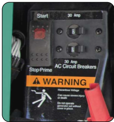
Generator main power & circuit breaker switches.
