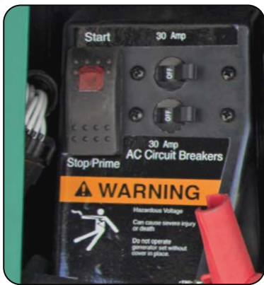
Generator main power & circuit breaker switches.
