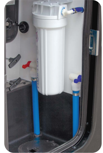
Low-Point Drains are located in the Universal Docking Station
