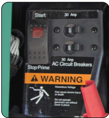
Generator main power & circuit breaker switches.
