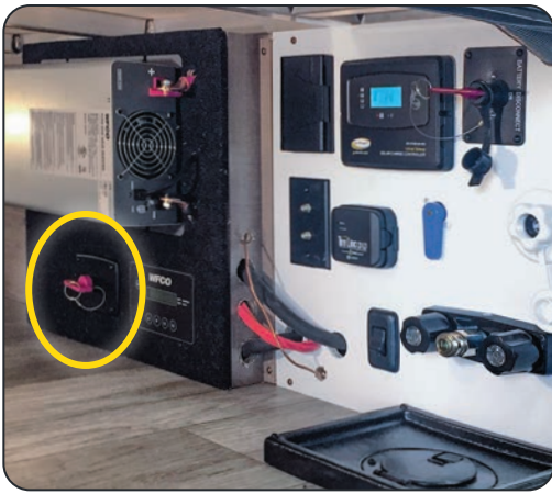
2000 Watt Inverter & 2nd Battery Disconnect
