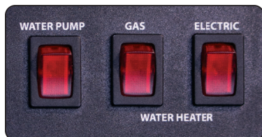
Water Pump & Water Heater On/Off Switches
