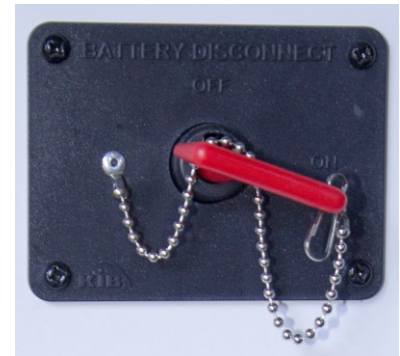
Typical battery disconnect switch
