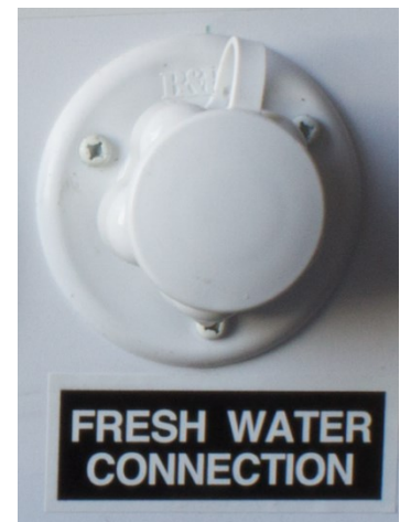
Typical city water inlet
